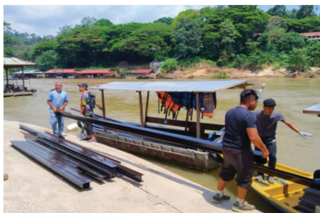
Fig. 2b. Materials for repairing damaged walking paths and the canopy walkway were transported to the sites by boats and then on foot.
